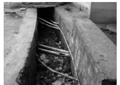
Part of the piped distribution system in Hubli
